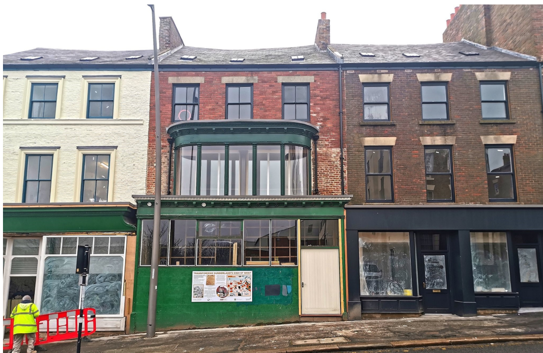
Restored street frontage nearly complete 170-5 High Street West, Sunderland Tyne and Wear Building Preservation Trust
